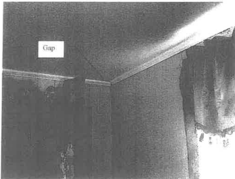
Photograph 6 – Molding Gap at Living Room Right Rear Corner
