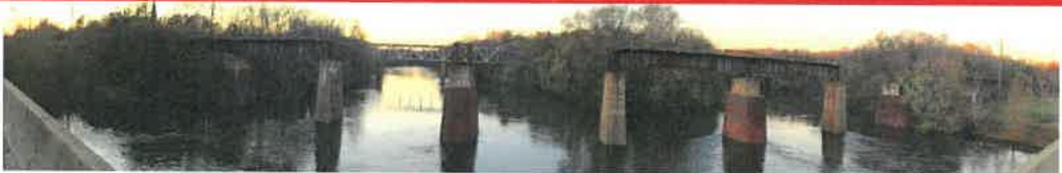
The existing Roanoke River bridge substructure is still intact and suitable to support the planned replacement Roanoke River Bridge.
