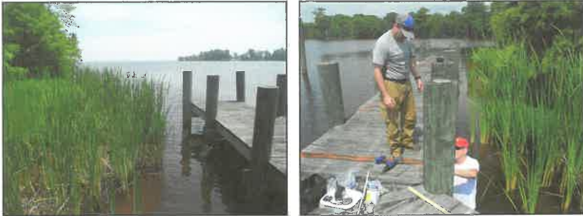
FIGURE 7. Left panel is looking east from the heavy duty dock located within the semi-protected waters at the mouth of Salmon Creek down the length of Albemarle Sound. Right panel is looking west up the Salmon Creek with the installation of a water-level recorder to monitor storm events.
